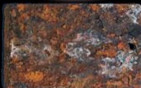
Control Panel (Unprotected Metal)
